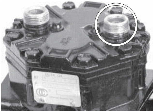
Stripped Fitting due to overtightening service valve.
